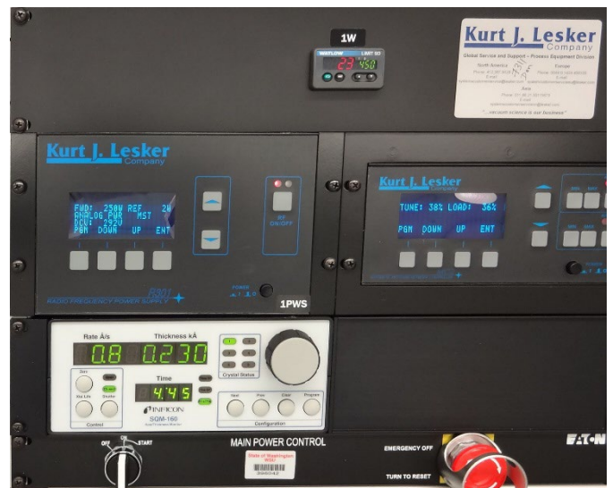
Figure 3 Controls including R301 & MC2 power control and SQM-160 film thickness monitor.
